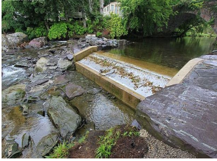
Coanda screen and intake
