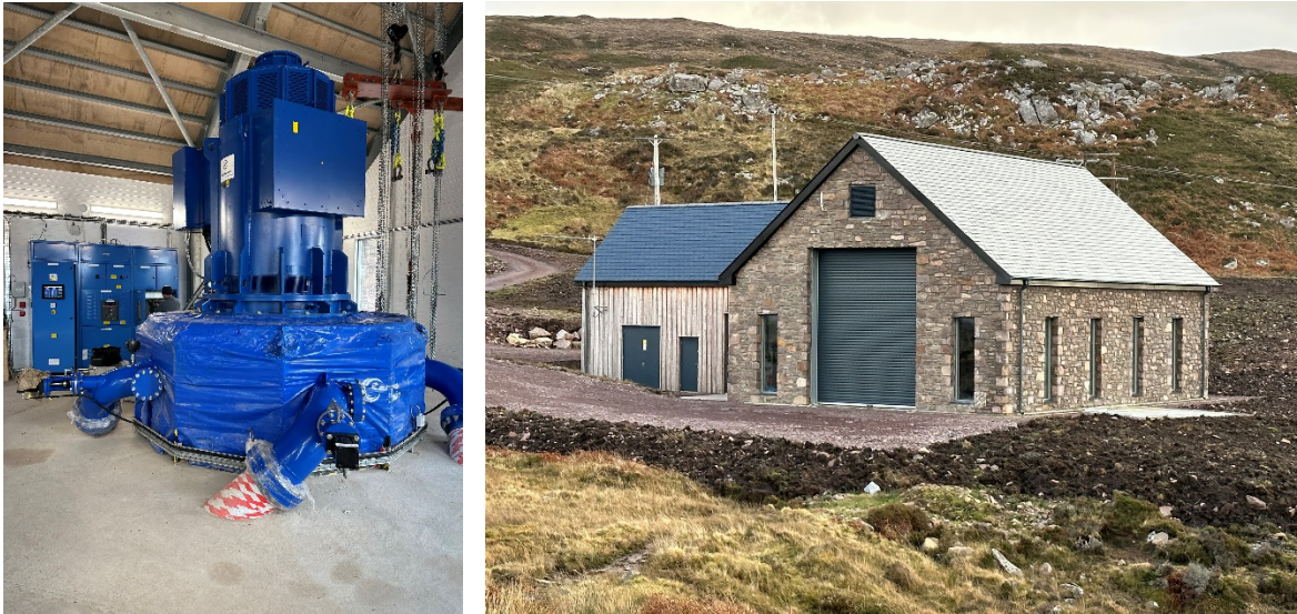
Figure 3 – Turbine and power house, a low visibility, low impact scheme that will generate for 100+ years (true energy security)
