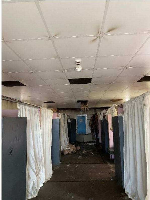
5. Smoke damaged dormitory to southern end of building
