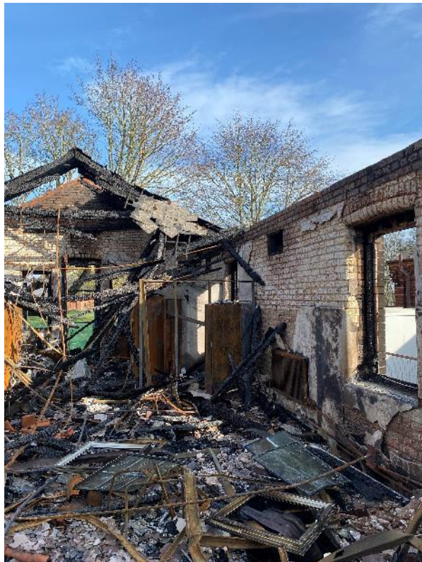
6. Internal view of fire damage (northern dormitory)
