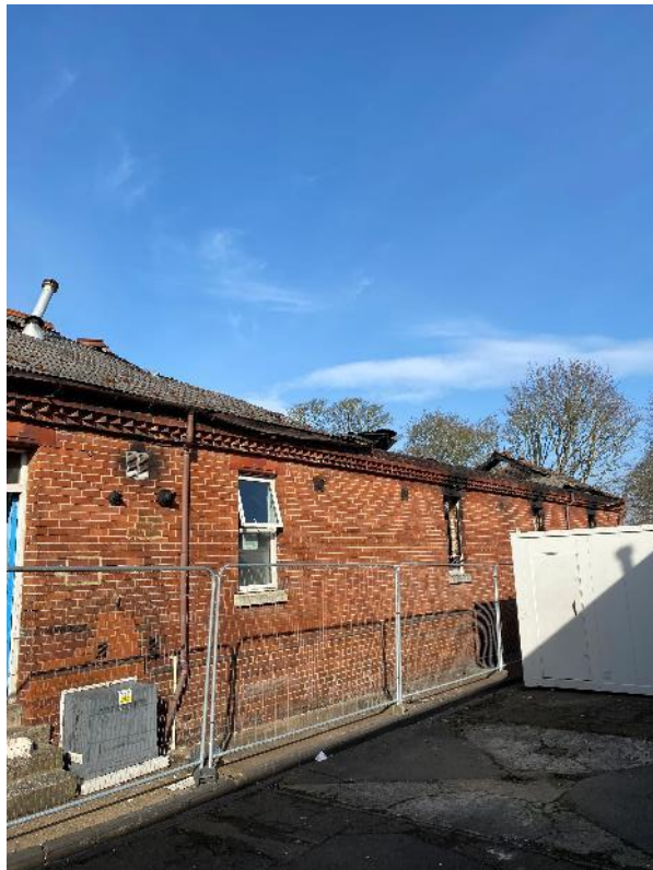
2. Right flank elevation (partial view of fire damage to roof)
