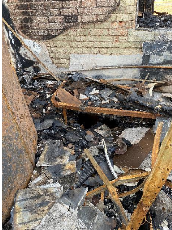
7. Debris in building with failed suspended timber floor beneath
