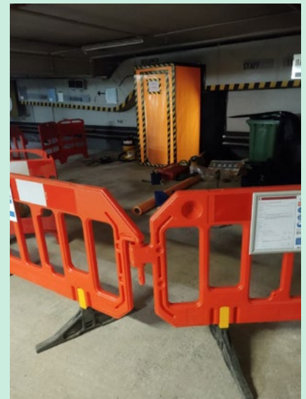
Walls and basement piles samples taken from Underground Car Park to help understand their condition
