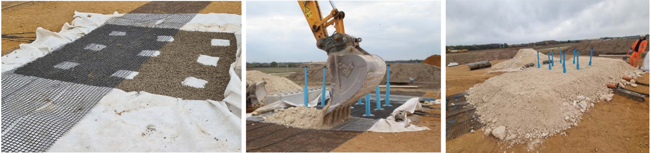
(c) Construction of site trial – Sensorgrid over water bags with backfill above
